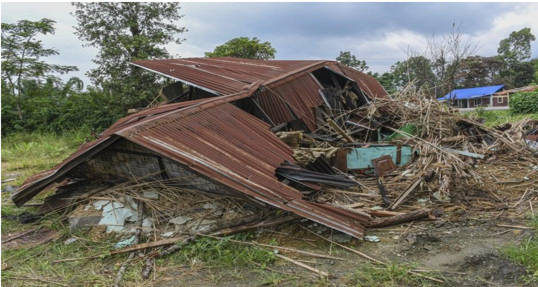
Figure 2: A destroyed house after conflict between Kukis and Meiteis along a highway in Torbung village in Churachandpur district, Manipur, May 3, 2023.
